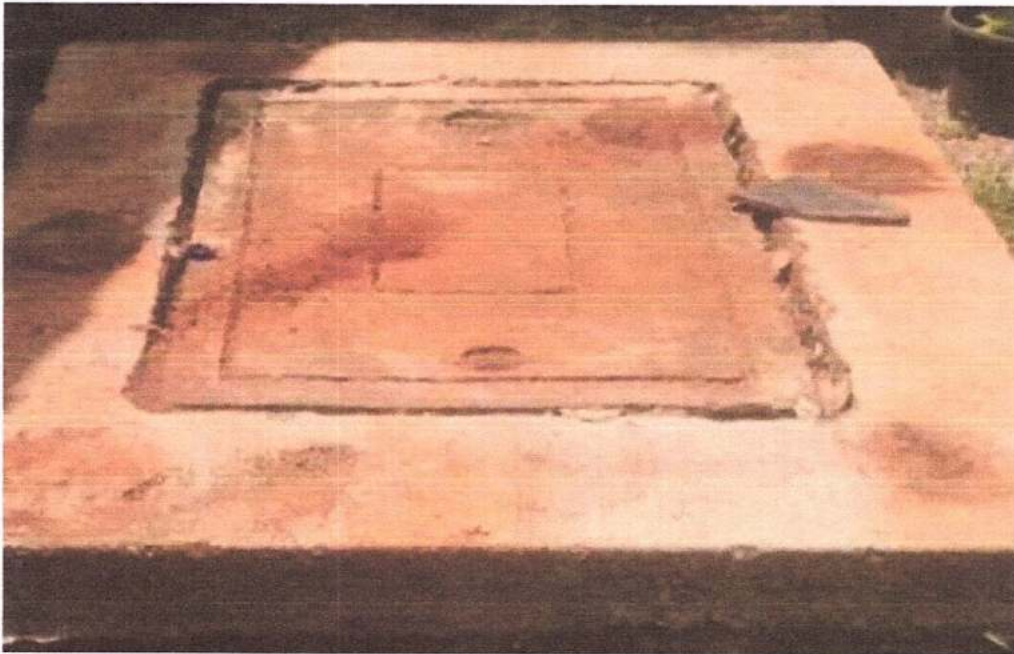
The Rainwater Harvesting System with ground water recharge has been installed
